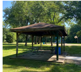
Picnic Shelter Fair condition
