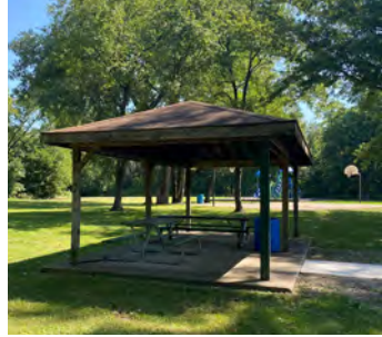
Picnic Shelter Fair condition
