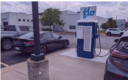
EV Charging Station - 531 Theater Rd
