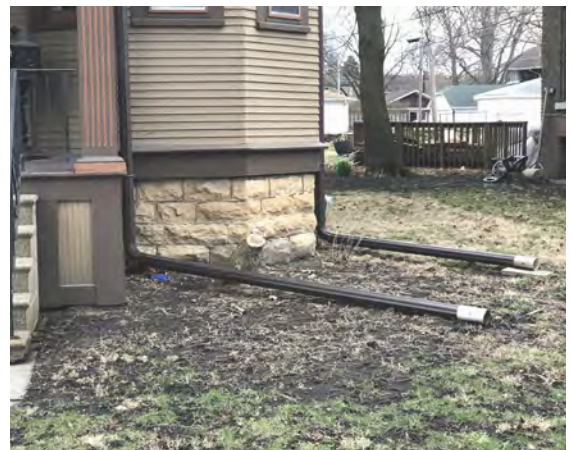
Locate downspouts away from significant architectural features to avoid water damage to the building. ✓
