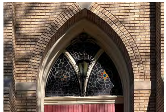
Identify areas of dirt, cracking, chipping, breakage, or missing glass. (314 E 8th St.)
