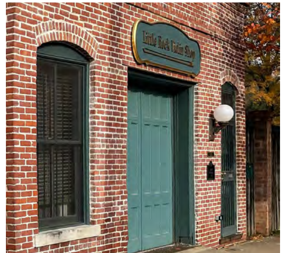
Provide regular maintenance of historic lighting to prevent deterioration. (316 E 11th St)
