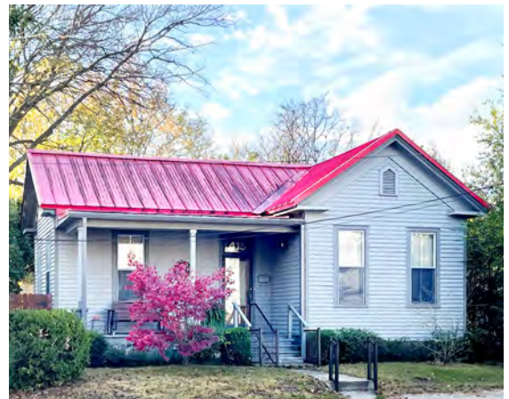
Provide physical or historical documentation when proposing a new roofing material. (415 E. 8th St.) ✓
